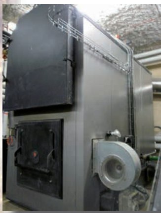
Chaudière Fröling LambdaMAT, 420 kW
